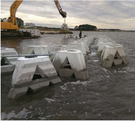
3.5-ft.-high WADs being installed to create a breakwater at the Seagrass Plantation Restoration Site in Delaware © Douglas Janiec
